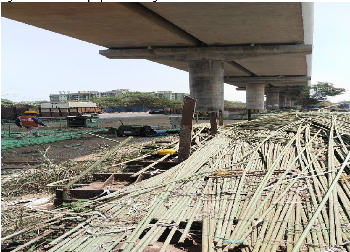
Figure 5: Haphazard storage of materials with rusted poles with sharp edges
