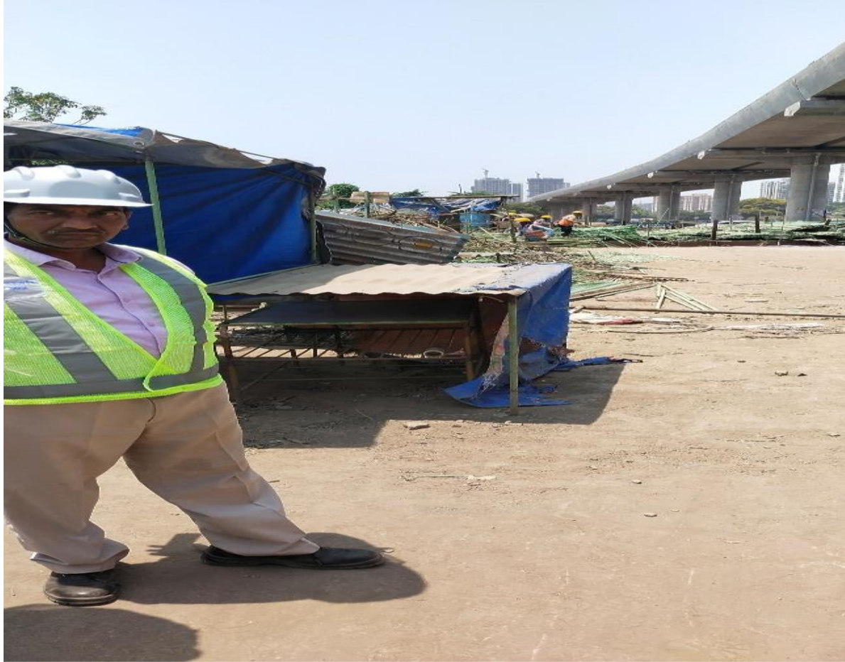
Figure 8: Work tables with corrugated sheets with sharp edges
