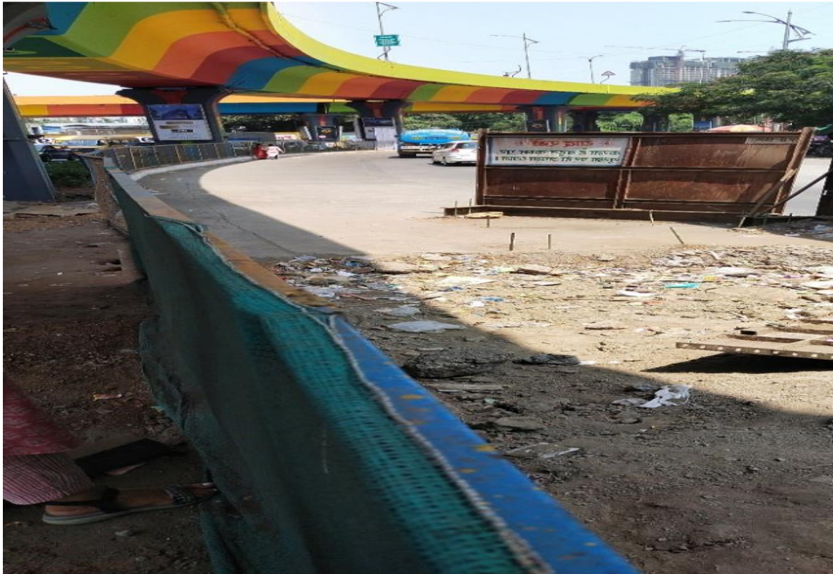
Figure 4: Partial and improper barricading of work sites
