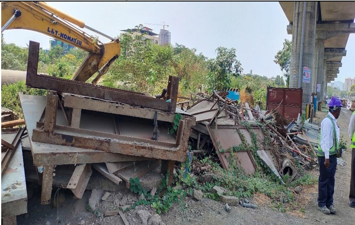
Figure 6: Haphazard storage of scrap materials
