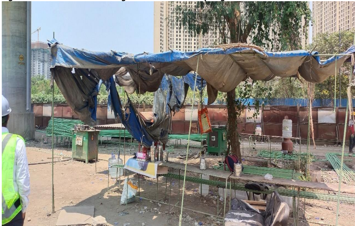
Figure 9: Poorly constructed worker lunch area with no facilities
