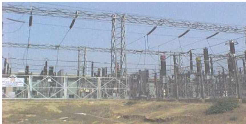
Typical High Voltage Receiving Sub-station
