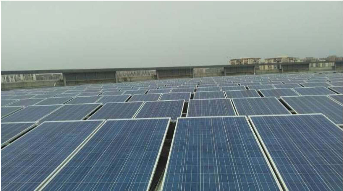
Solar PV Power panel
