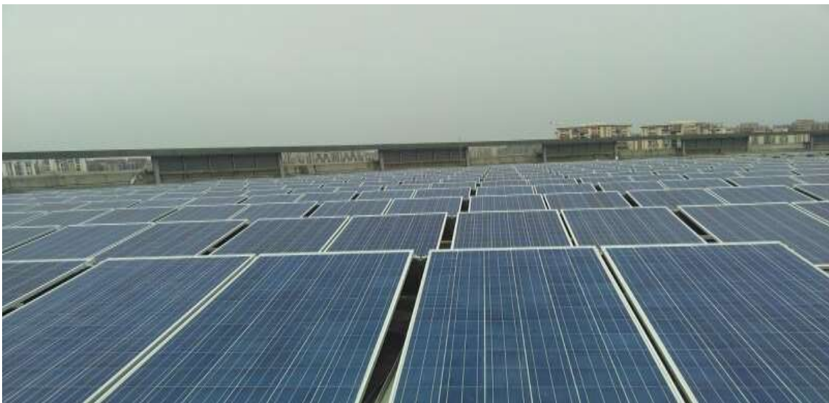
Solar PV Power panel
