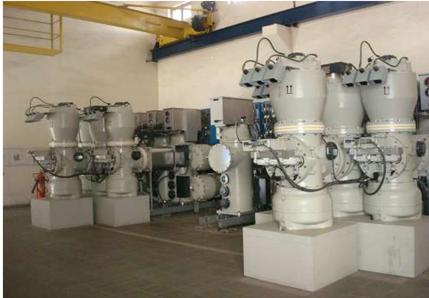
Typical High Voltage Gas Insulated Sub-Station (GIS)
